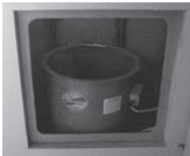
... machinery space ventilation and mud pit exhaust...
